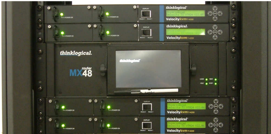
Figure C4: Rack-Mounted Router with touch screen mounted in a rack along with Thinklogical® VelocityKVM T-4200 units.
